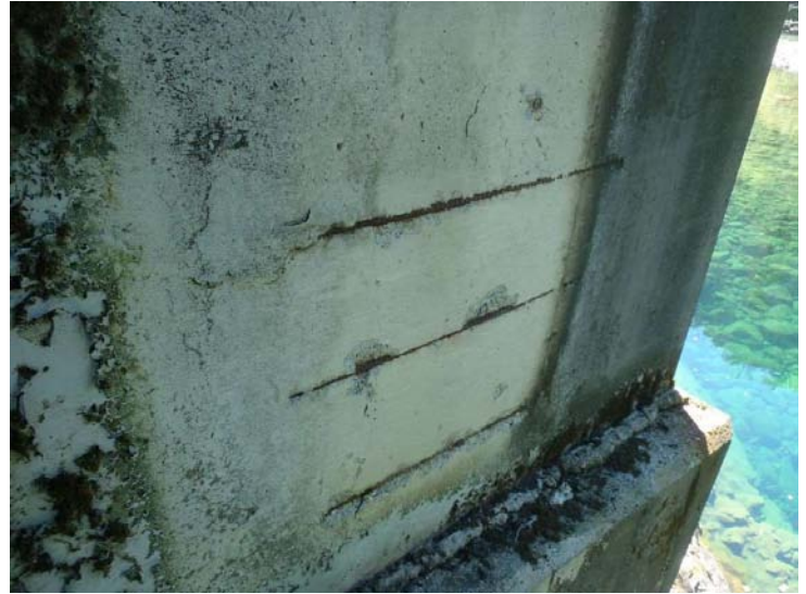
Photo 44: Pier 1 Right Face Exposed Reinforcing
