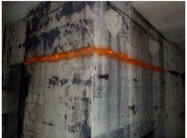
Photo 24: Span 2 Girder 2 at Pier 2 Full Width End Split
