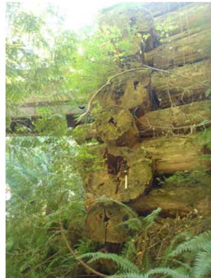
Photo 40: Typical Core Rot in Crib Face Log
