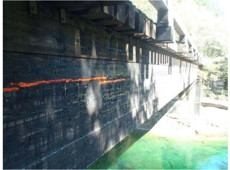
Photo 26: Significant Check AE251-AE280
