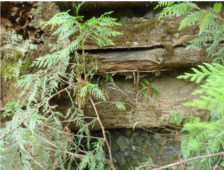
Photo 33: Left Abutment Downstream Wingwall Wide Split in 2nd From Bottom Log and Minor Scour
