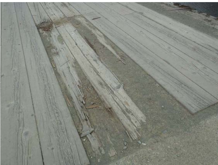
Photo 11: Typical Wear/Deterioration in Centre Running Planks
