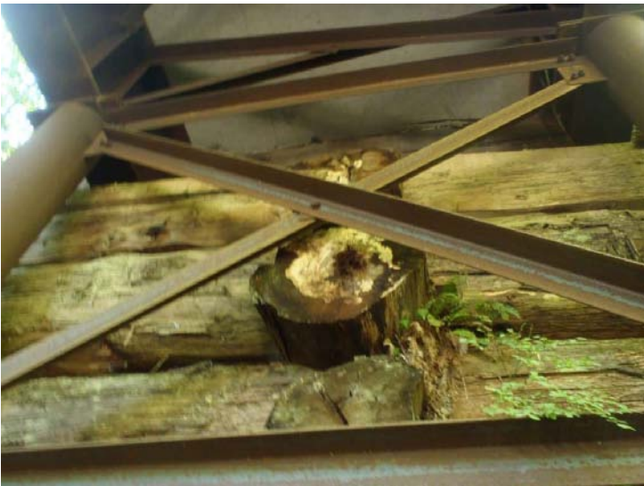
Photo 41: Right Abutment Fungal Growth On Tiebacks
