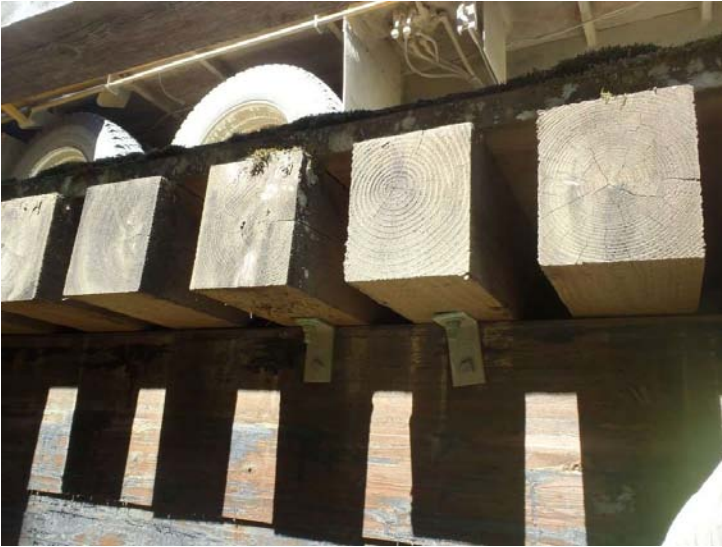
Photo 13: Typical Tie Condition
