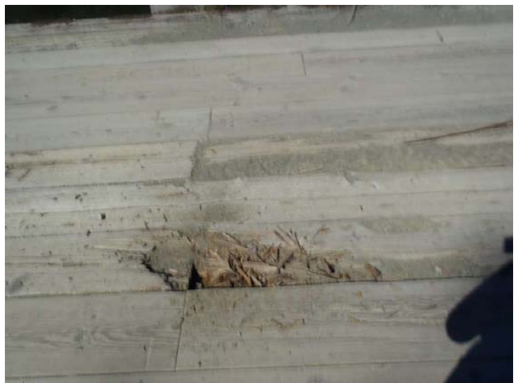
Photo 12: Pocket of Rot in Centre Running Planks
