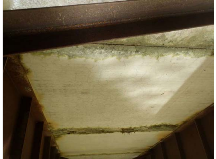
Photo 14: Typical Light Map Cracking on Underside of Concrete Deck
