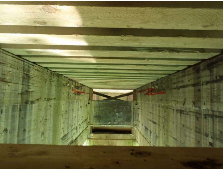
Photo 23: Span 2 Diaphragm 1 at Pier 1 Note Checking in Top Flanges Of Girders 2 & 3
