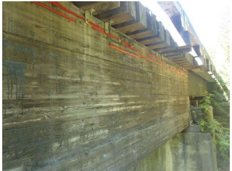
Photo 22: Span 2 Girder 1 Upstream Face Top Flange Series of Checks Along Whole Length
