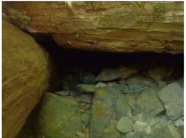
Photo 34: Left Abutment Downstream Wingwall Minor Scour
