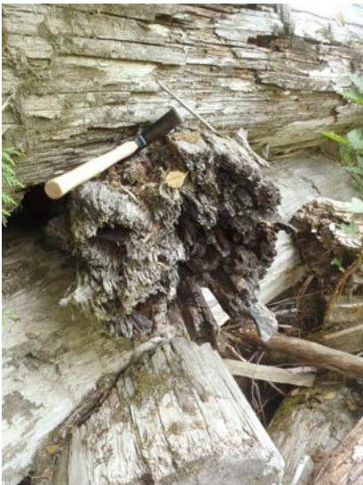
Photo 35: Left Abutment Downstream Corner 2nd Tieback From Bottom End Rot
